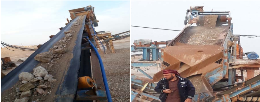
Photo 3. The demolition waste subbase on the belt of crusher and sieve process after crushing.
