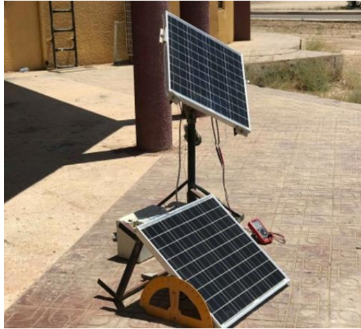
Figure 7. Multi-axis solar tracker and static solar panel
