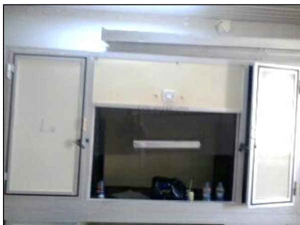
Figure (1): Fume hood installed improperly in one of the chemistry laboratories with poor quality and inefficient ventilation system
