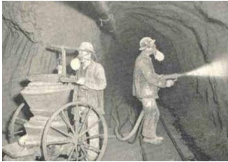
Figure 2-1 Lining a tunnel with Guniting using a double-chamber gun during the 1920s [32]
