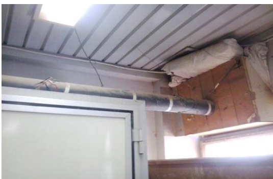
Figure 2: Incorrect installation of gas and vapours tubes which may lead to leakage.
