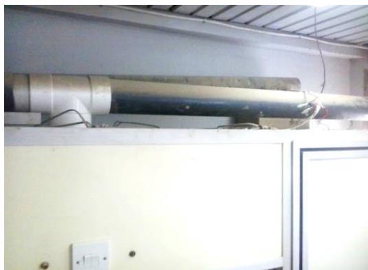
Figure 1: Improperly installation of fume hood can make a number of risks to postgraduate students.
