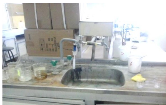
Figure 5: Connections, water pipes and pipes from materials not complying with laboratory specifications.
