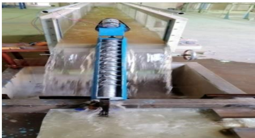
Fig. 5. Archimedes screw with hydraulic channel during operation
